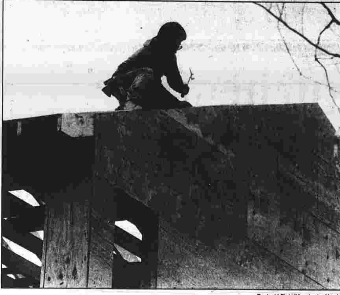
NAILING IT DOWN — Rennie Sumera of Pomfret works recently atop a house under construction at Hickory Lane and Butterworth Road.
